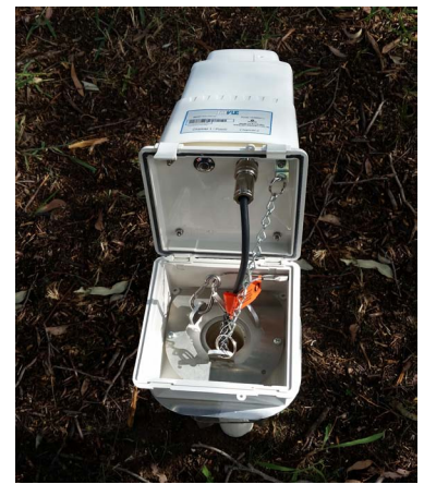
Submersible Level / Pressure sensor attached and lowered into the bore well.
