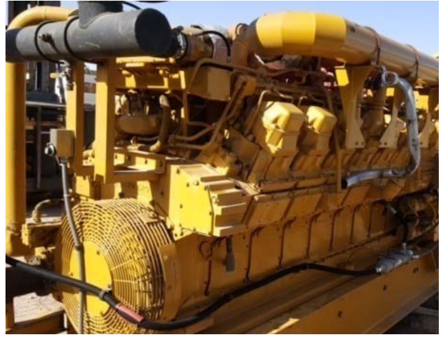
Remote monitoring and alarming ensure asset protection
